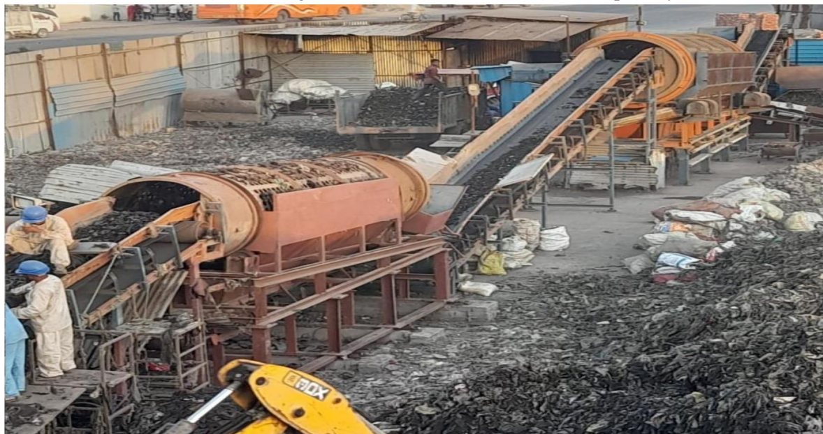
Fig.4 Existing Trommel machine installed in Rudrapur city
