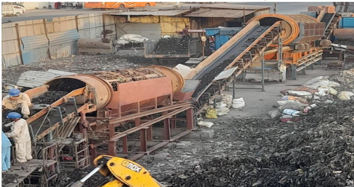
Fig.4 Existing Trommel machine installed in Rudrapur city
